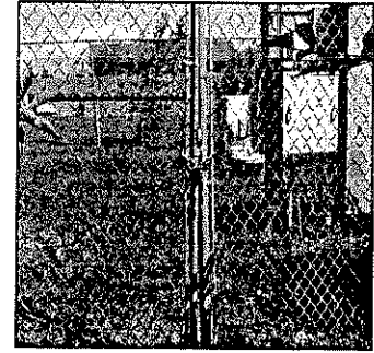
Fig. 4 – Secured well lot with Willow well head and misc. electrical panels.
