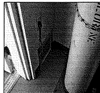
Fig. 6a – Chlorination room associated with the 1 mg. storage tank.
