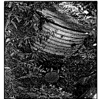
Fig. 1 - Spring collection area showing overflow pipe.
