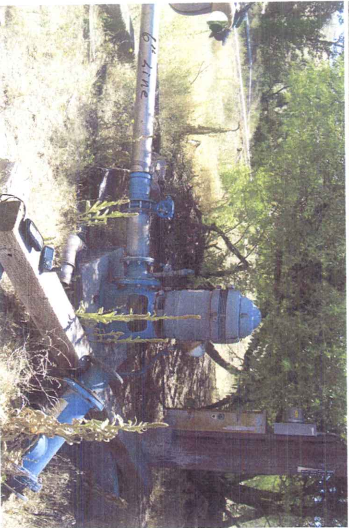
Well + Pump 20 HP.
