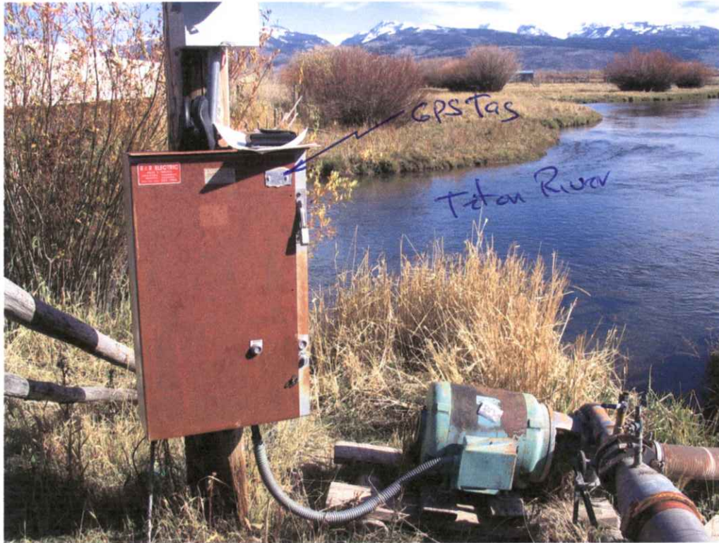
A22-00587 - Relift pump (v2/diversion)
