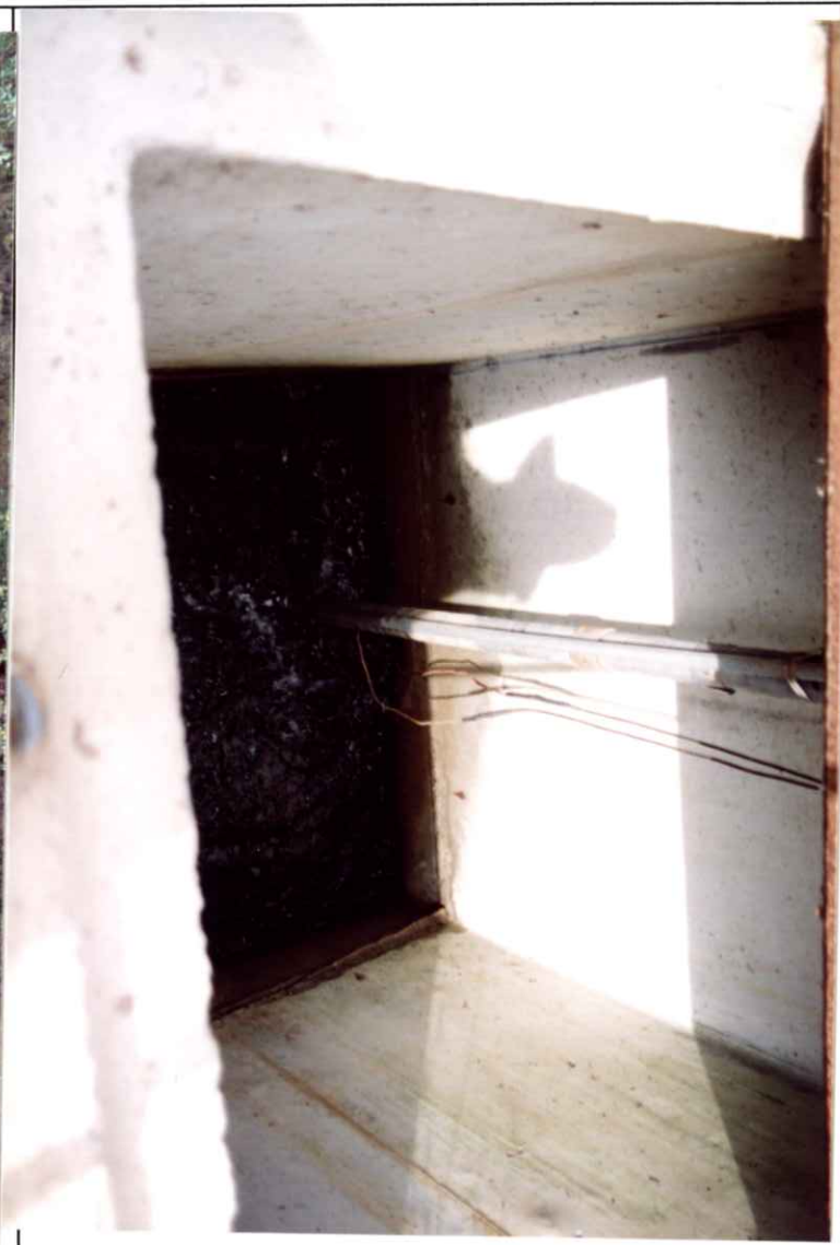
⑤ Inside pump vault @ laypoint 24 9 Sept 05
