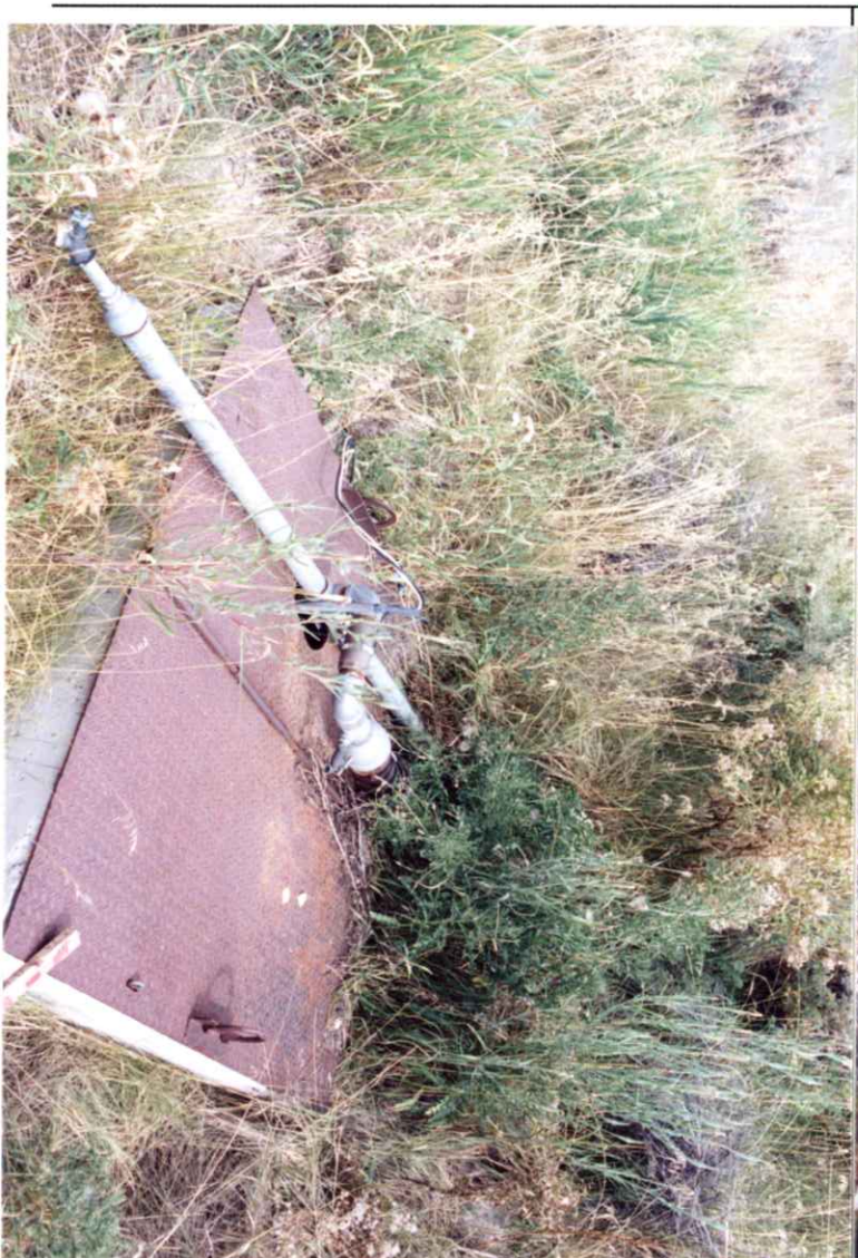
④ Pump vault @ Waypoint 24 9 Sept 05
