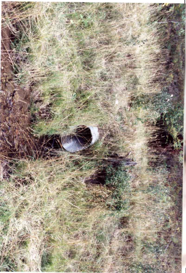
⑥ Over flow from pipe inlet laypoint 25 9 Sept 05 Bce
