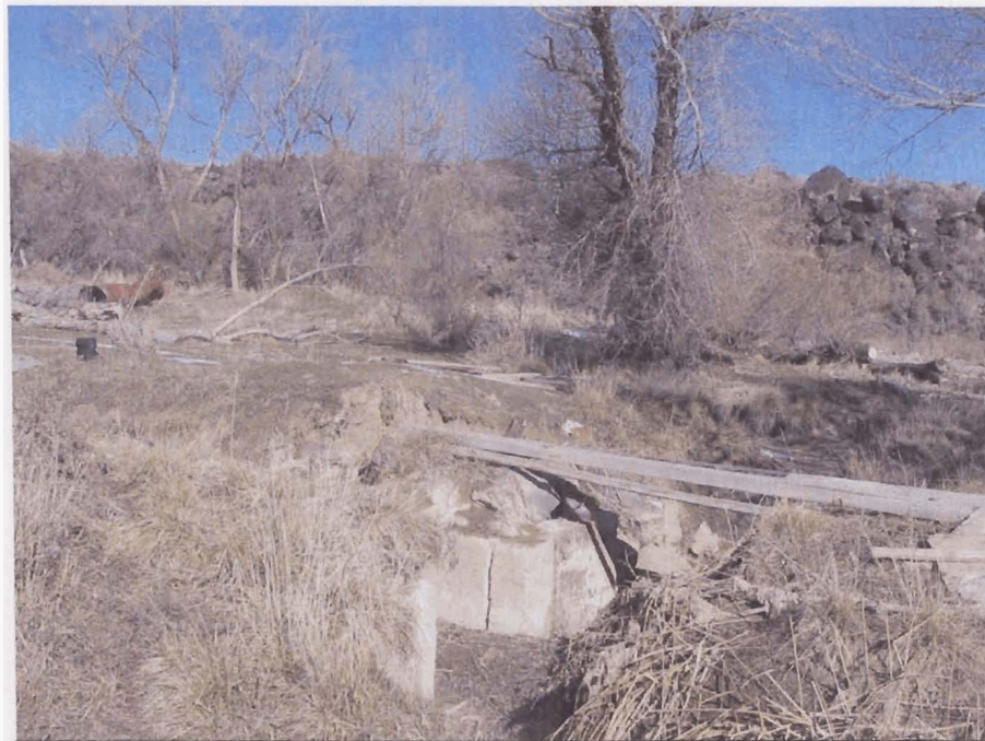
Photo 468 Gene1. Looking down stream mostly North-Northwest. Tag A0016122 10S, 18E Sec 3 SWSWSW
