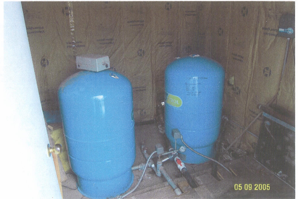
Inside Cold Water well pump house
