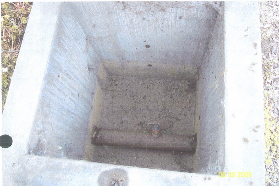
One of Two Flow Meters measuring Hot Water Well discharge
