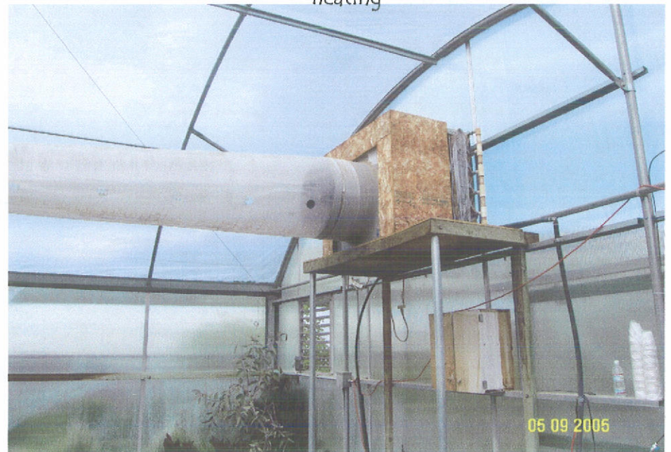
Hot water Heat Exchanger for Green House heating
