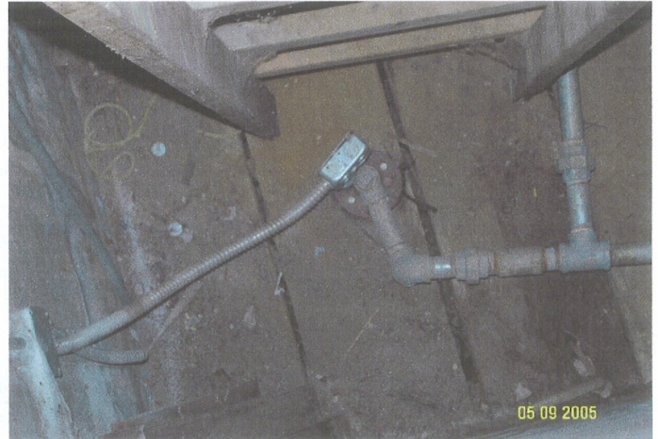
Well / Pump Head 6" well - 1.5 HP
