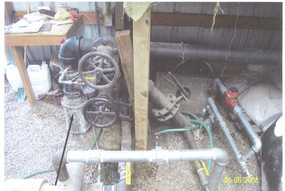
Hot water Artesian Well head
