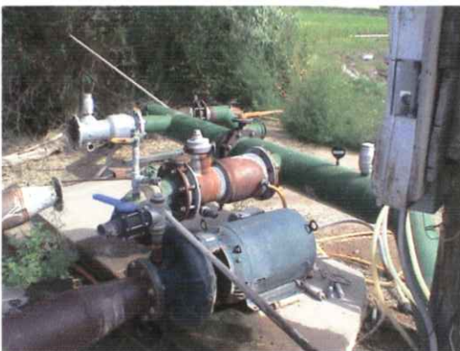
Main Motor and pump at POD.
