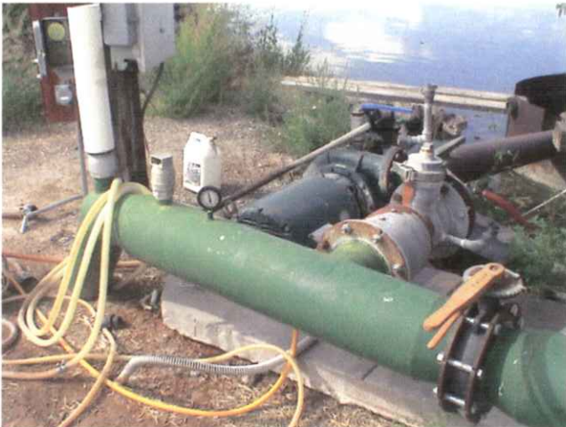
Pump and Motor: Main line to west fields.
