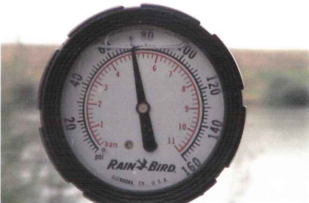
Pressure at pump.
