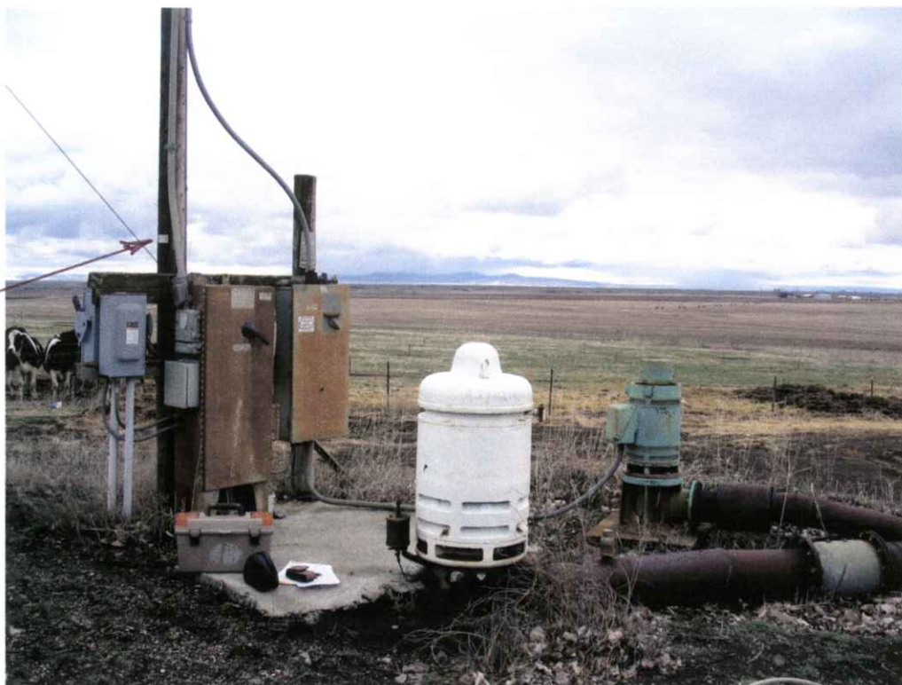
A21-2110A+B - Well, pump + booster, looking East
