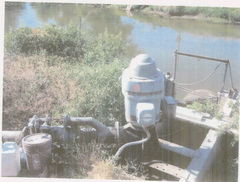
River Pump (Blackfoot River)
