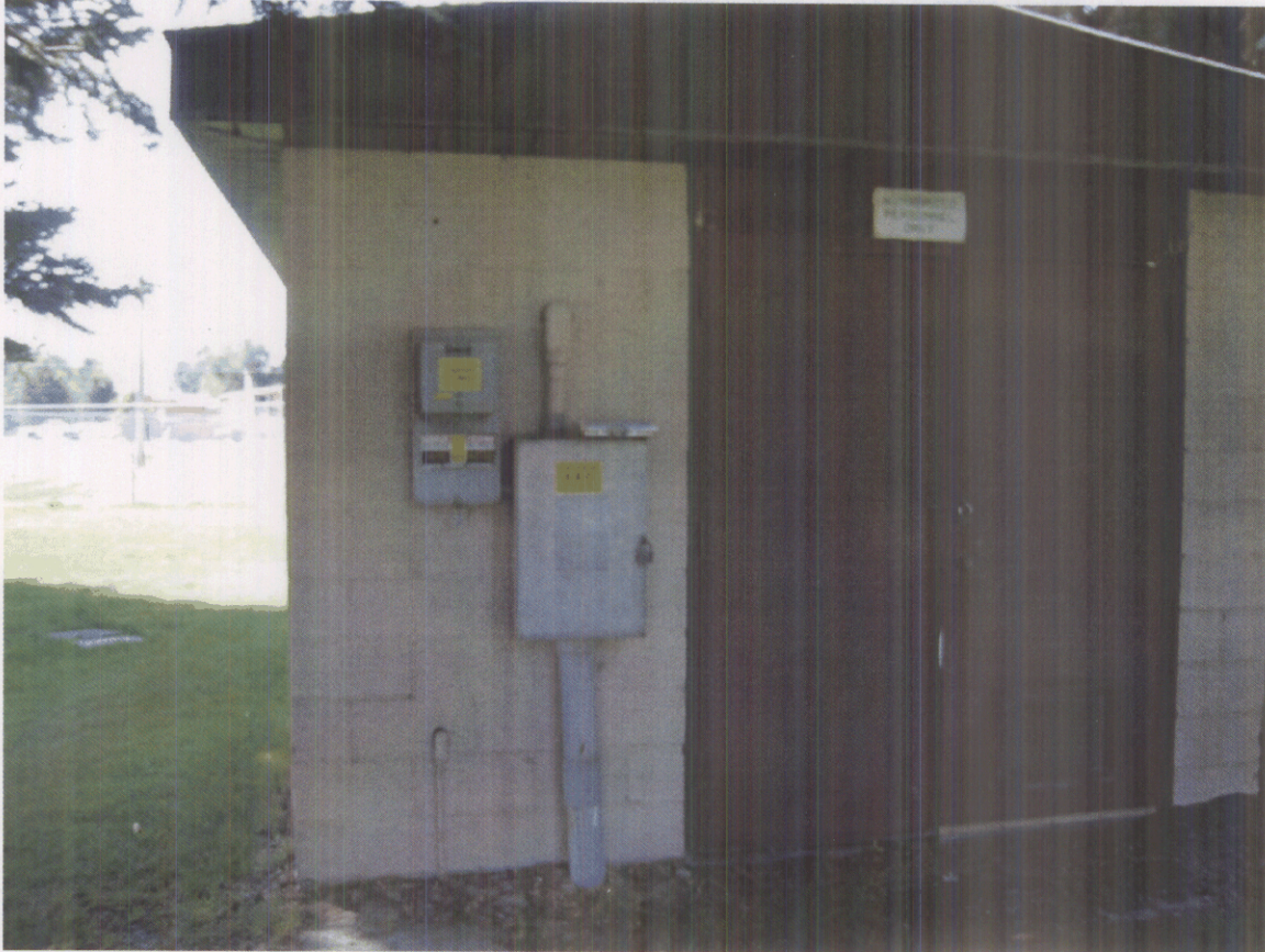
Looking West at Point of Diversion pump house. Well located in the pump house and sits in the public park with horseshoe pits just south of pump house (csaxton 8/7/02).
