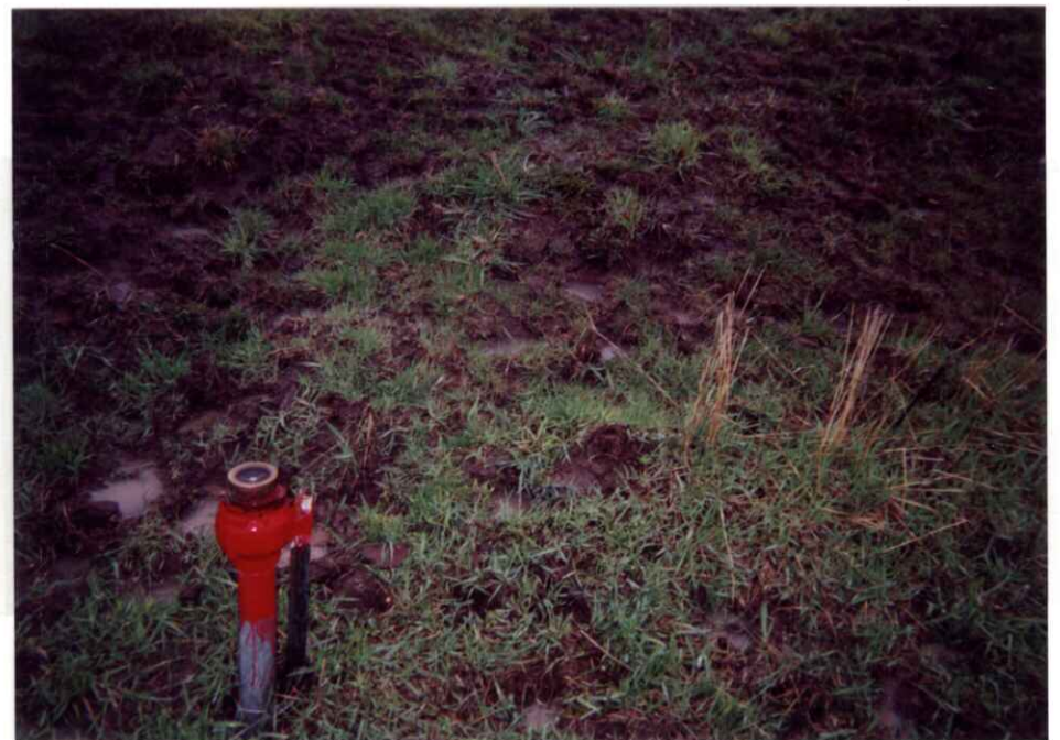
1 of 35 underground sprinkler heads
