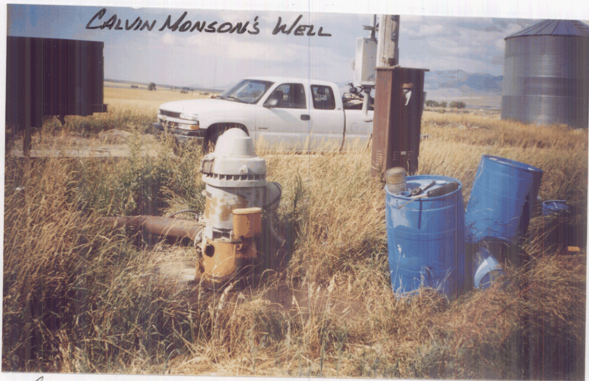
CALVIN MONSON'S WELL. DISCHARGES TO MAINLINE FOR SPRINKLER IRRIG.
