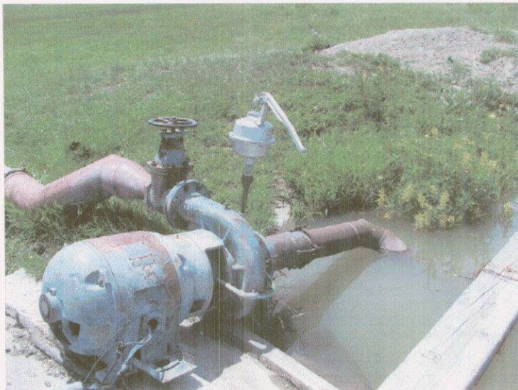
Photo 8. Close-up of the 30 hp pump for Toponce water.
