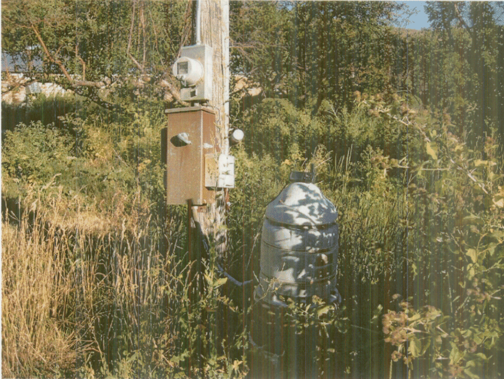
Looking North at main irrigation well. Claimed POU surrounding well. Hp = 10 (csaxton).
