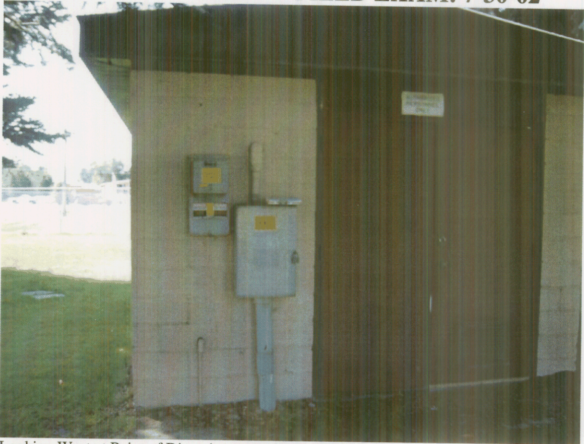
Looking West at Point of Diversion pump house. Well located in the pump house and sits in the public park with horseshoe pits just south of pump house (csaxton 8/7/02).
