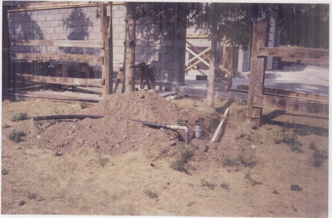
Headend and Irrigation System put in place July 2002 to replace Historical System.
