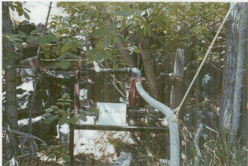
Looking West. Pump from Portneuf. Portneuf behind me in picture.
