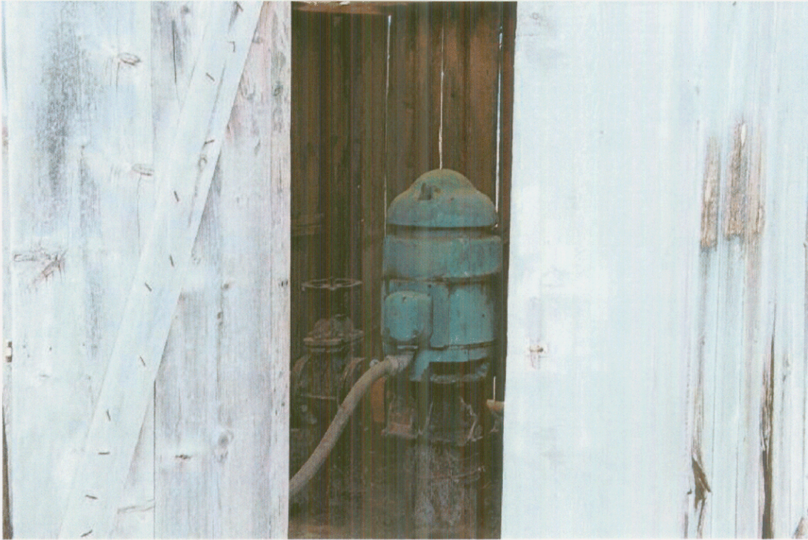
Irrigation well inside well house (csaxton 10/24/01).
