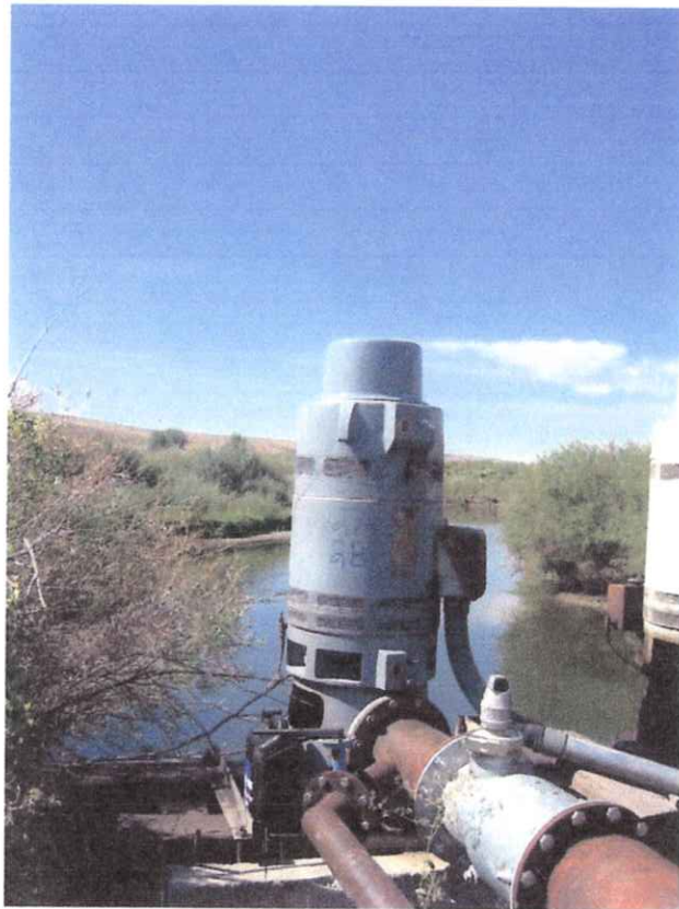
200 HP River Pump (Blackfoot River)
