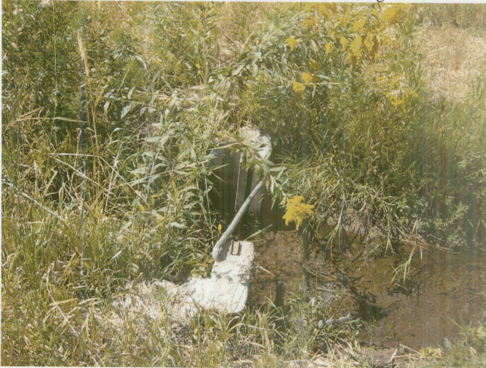
Looking at a headgate in the ditch to divert water to claimed POU (csaxton)
