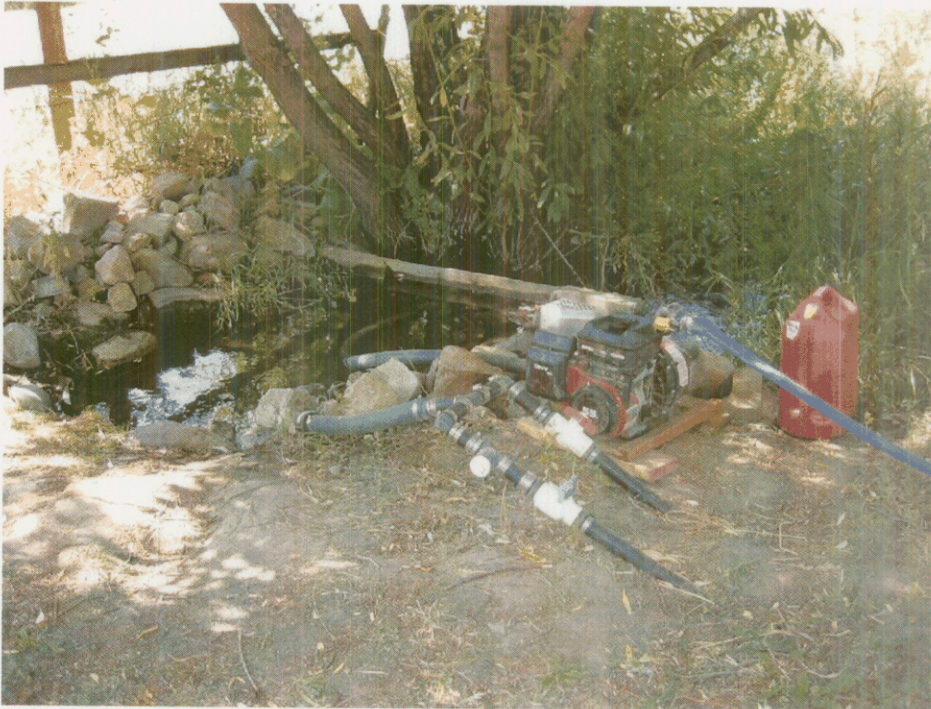
Pump that diverts water from the ditch system. Not an actual POD since it is diverting from a ditch (csaxton).
