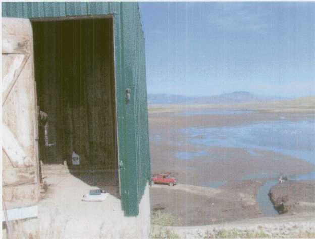
Photo 4. Release gate at Chesterfield Reservoir.
