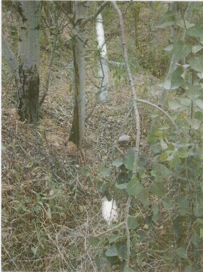
Looking East. Pipeline that delivers water to claimed POU (csaxton).
