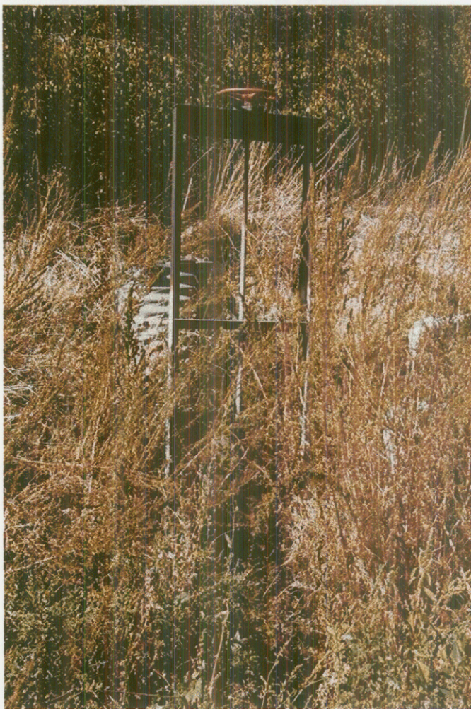
Looking West. Intake line for pump drops into the corrugated metal pipe. Valve can restrict outflow of the creek (csaxton 10/5/01).
