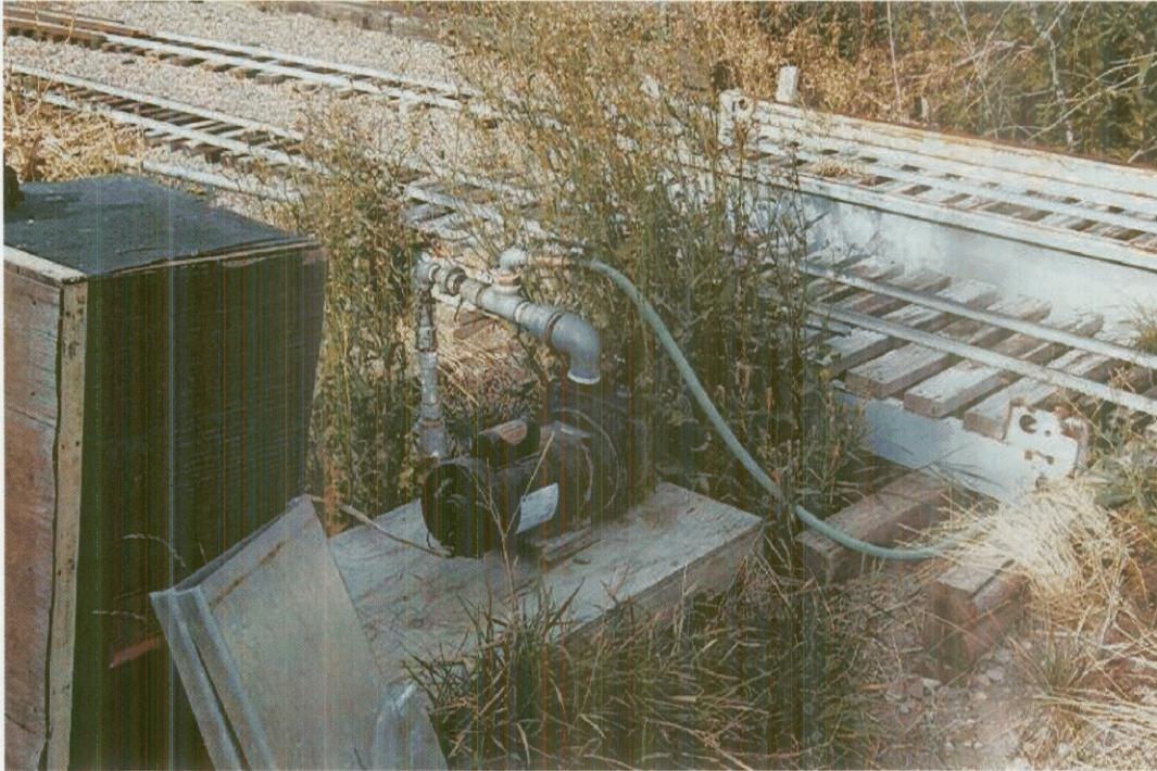
Looking NW. Pocatello creek on the other side of the RR tracks. Pump outflows to a 2 in underground PVC to sprinkler system. Pump is a Magnetek – Centurion. 1.5 hp; # 7-164300-24; AMPS SF 9.2/18.4. (CSAXTON 9-25-01)
