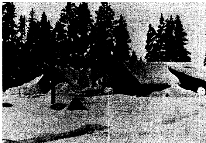
Heavy snow at Mack's Inn meant a lot of shoveling to get the weight off the roof! Quite often a wire was used to slip the snow - a neat trick!
