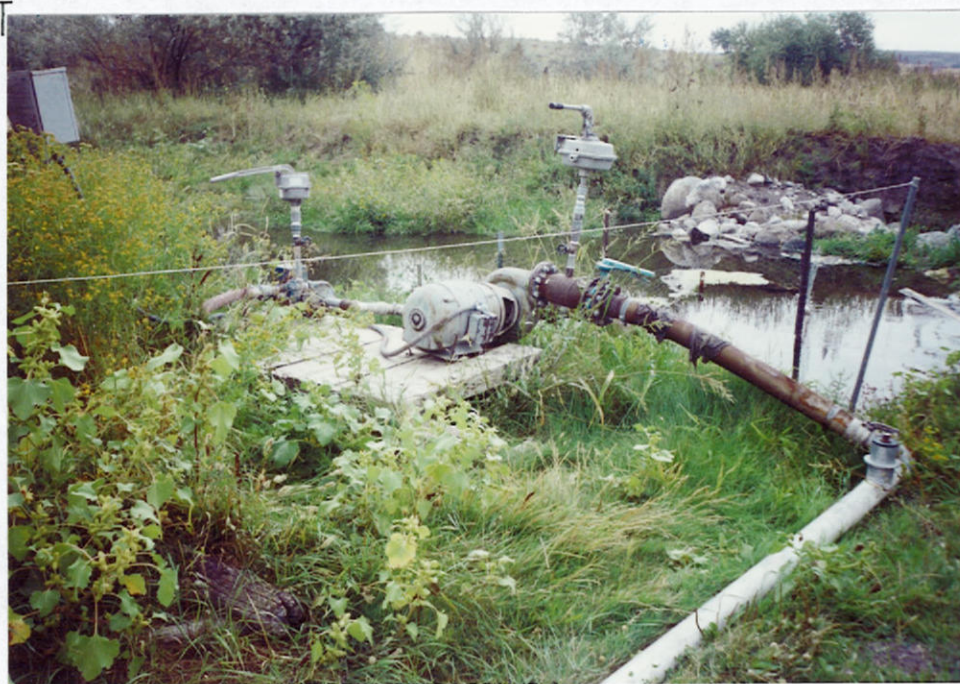
Photo #3 Looking SE from the SWNW NW of Sec 36 T55R9E Showing 2 pumps, taking water from Little Canyon Creek. The smaller is for domestic lawn & garden and the larger is for irrigation
