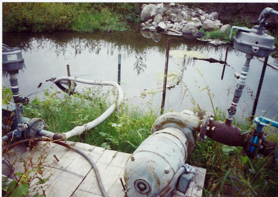
Photo #4 Looking SE from the SWNW NW of Sec 36 T55R9E Showing 2 pumps taking water from Little Canyon Creek. The smaller is for lawn and garden and the larger is for irrigation. See attached notes for pump specs.
