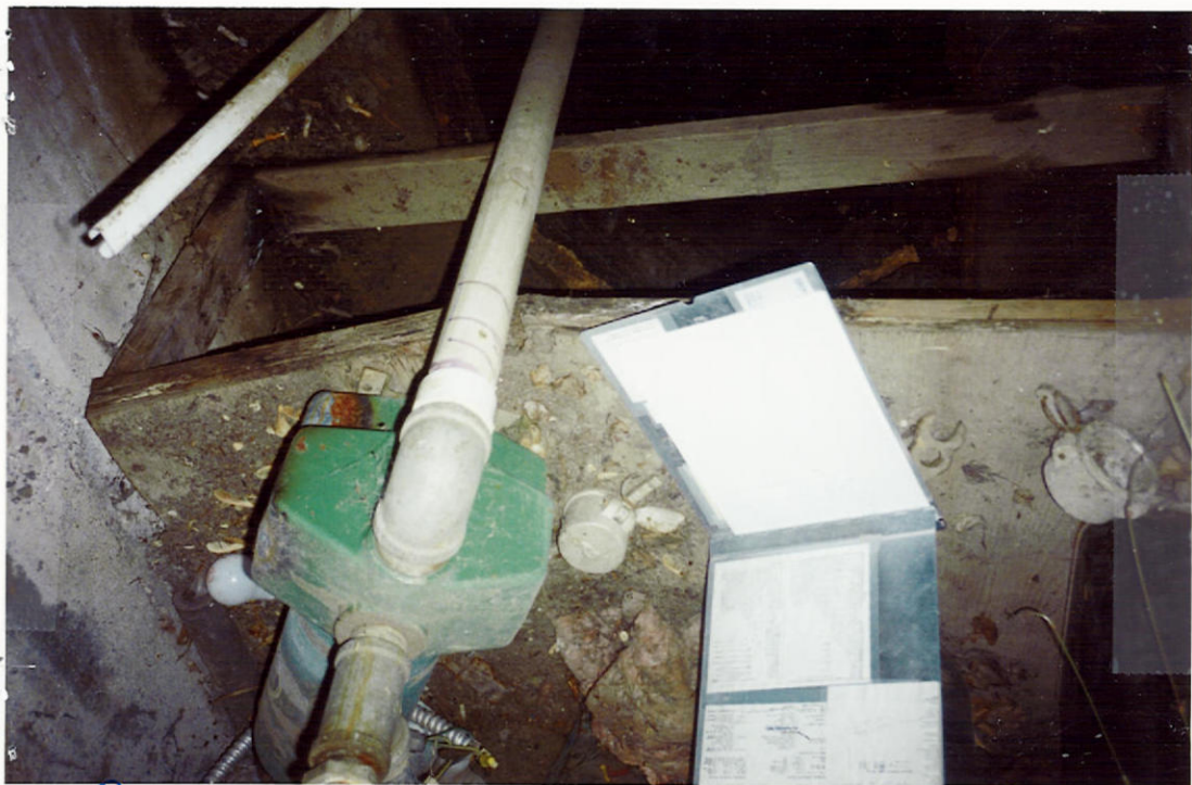
① Point of diversion. Well is open hole, covered by secure well house 2.4' diameter 12' deep
