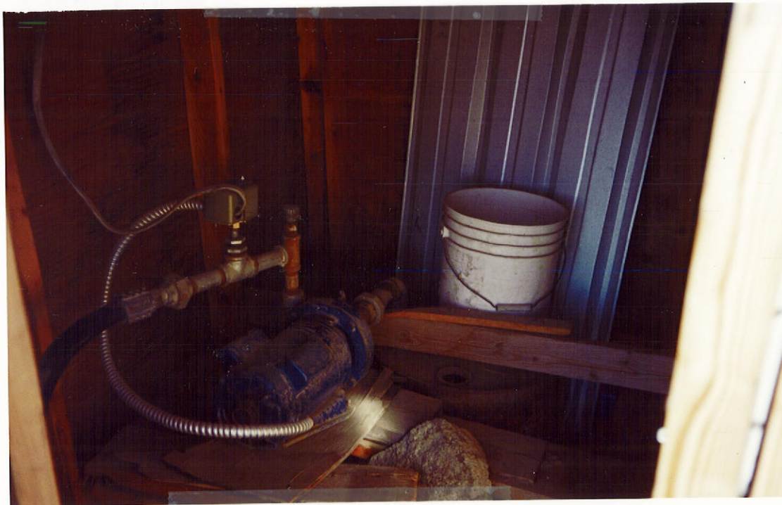
Photo #1-4 Looking SW into Pump house showing Pump #2
