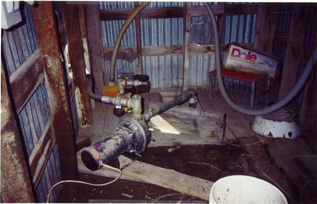
Photo #1-3 Looking S into Pump house showing the Pump #1
