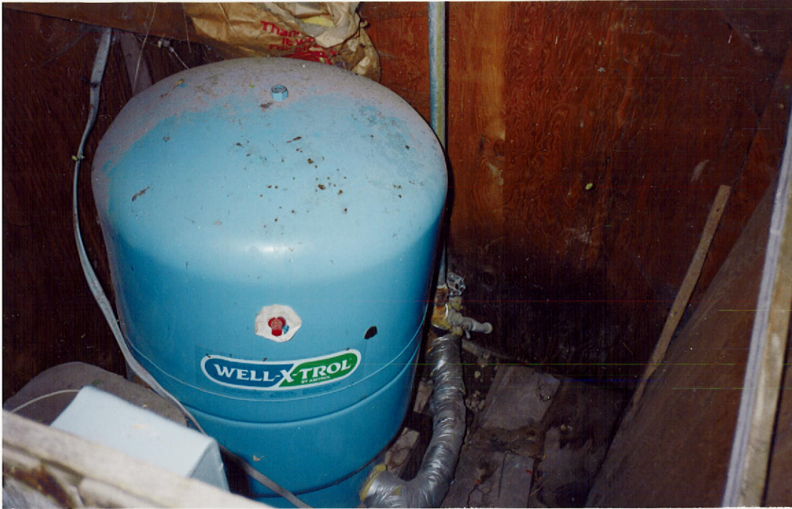
Pressure tank located in well house of well drilled in 1961 T03S R06E S11 SWNW SW
