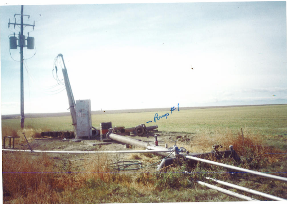
Photo #3 10-23-86 Looking SW from the SE NW NE corner of Section 32 showing Pump #1 which has been pulled for maintenance
