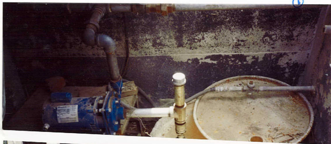
① Well No. 1 NWSENE On east side of property Cement casing
