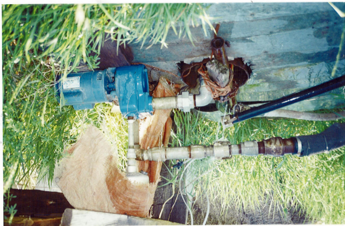
① Point of diversion. Open 12" casing with 2 HP pump. Toss rock S. 36 NWS 5W
