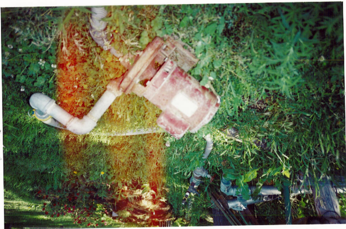
② Booster pump for garden plot
