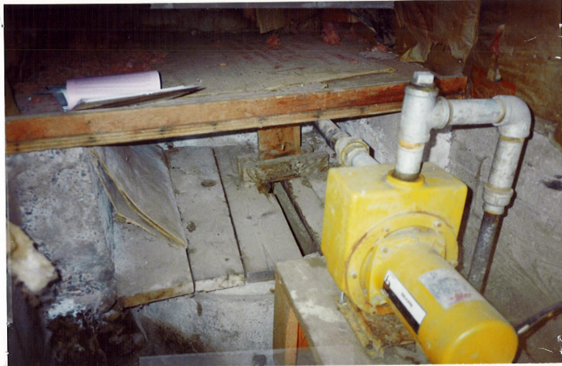
① Well & pump T033 R06E S.36 SESENW
