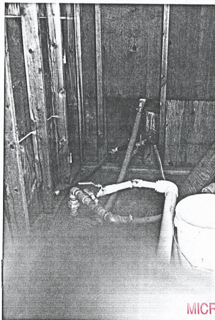
PICTURE # 2. SHOWS INSIDE OF WELL HOUSE.
