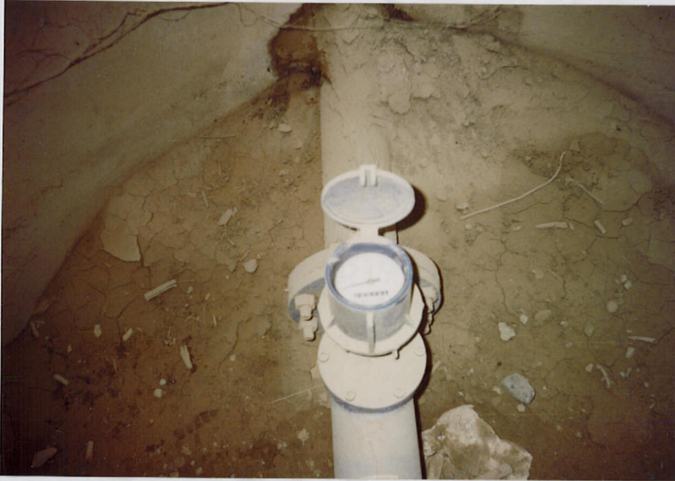
Well meter on well dating from the 1930's. Well access is through a manhole cover in lot behind Homedale City Hall.
