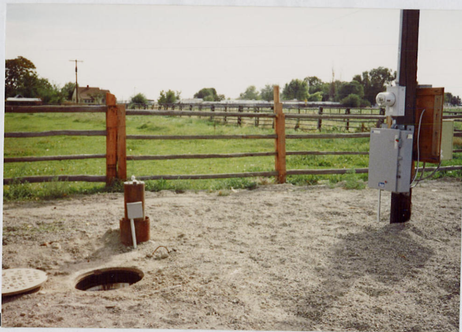
New well casing, access and power supply. Well is on 1st St., approximately three blocks south of Homedale City Hall
