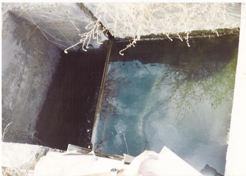
2-way concrete irrigation box
