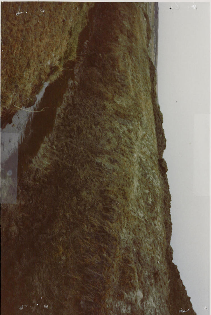
Drain with spring water in it.
