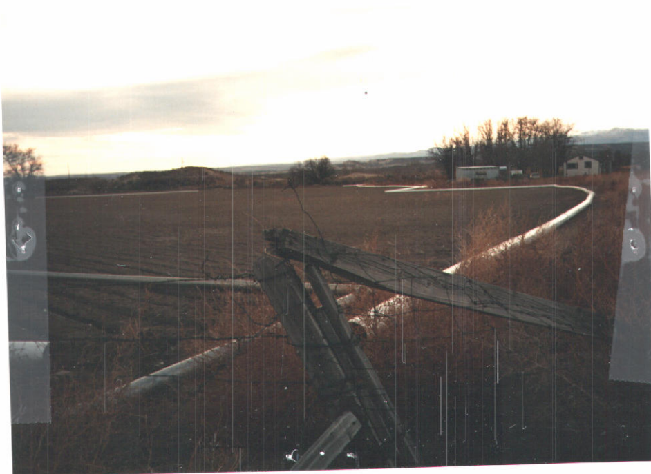
Gated Pipe in western Portion of field. Pictures 4&5 taken on 11-29-90.
