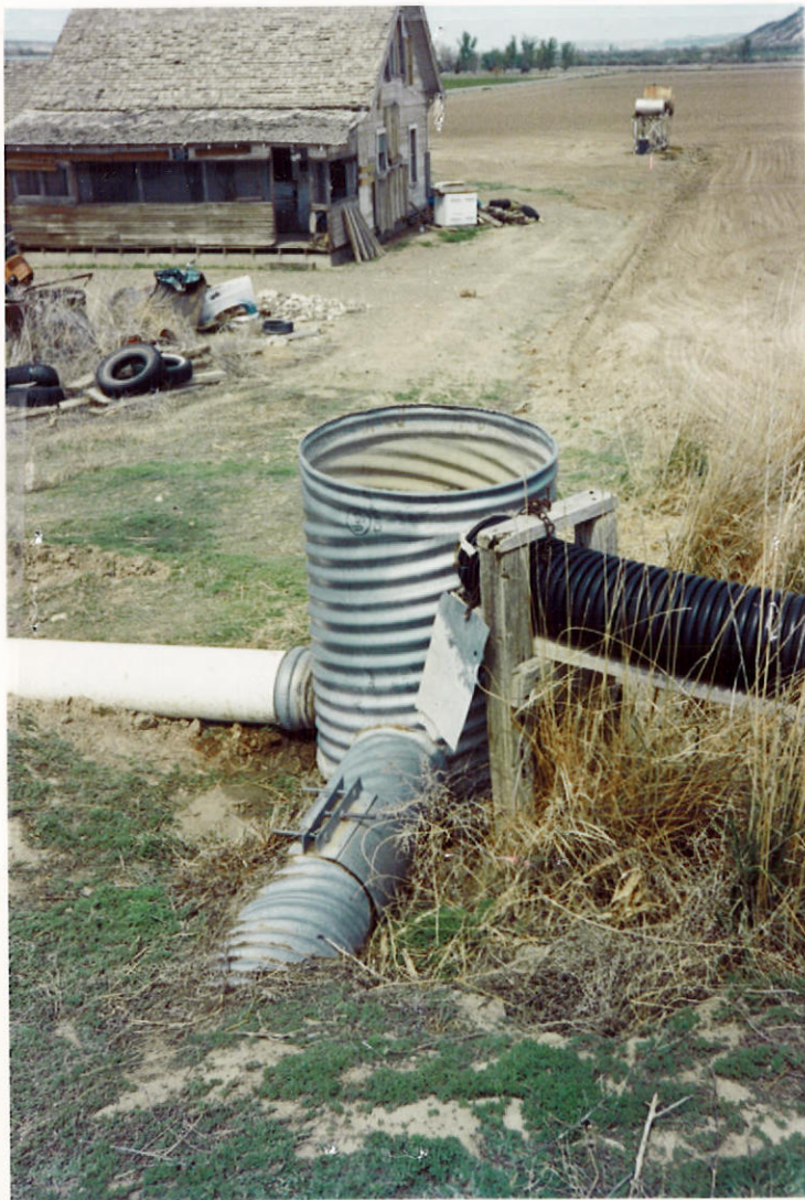
This is the intake point of the irrigation district water. Conveyance is by Gravity Flow Pipeline.
