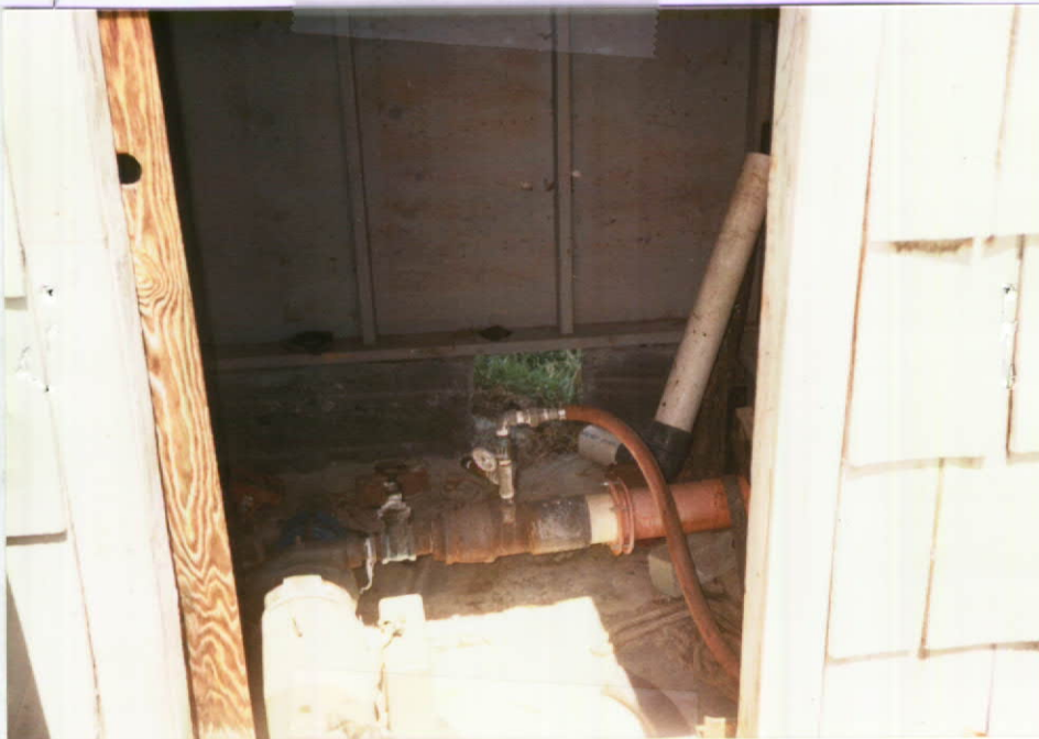
Pumphouse w/ 1/2 hp pump from pond
