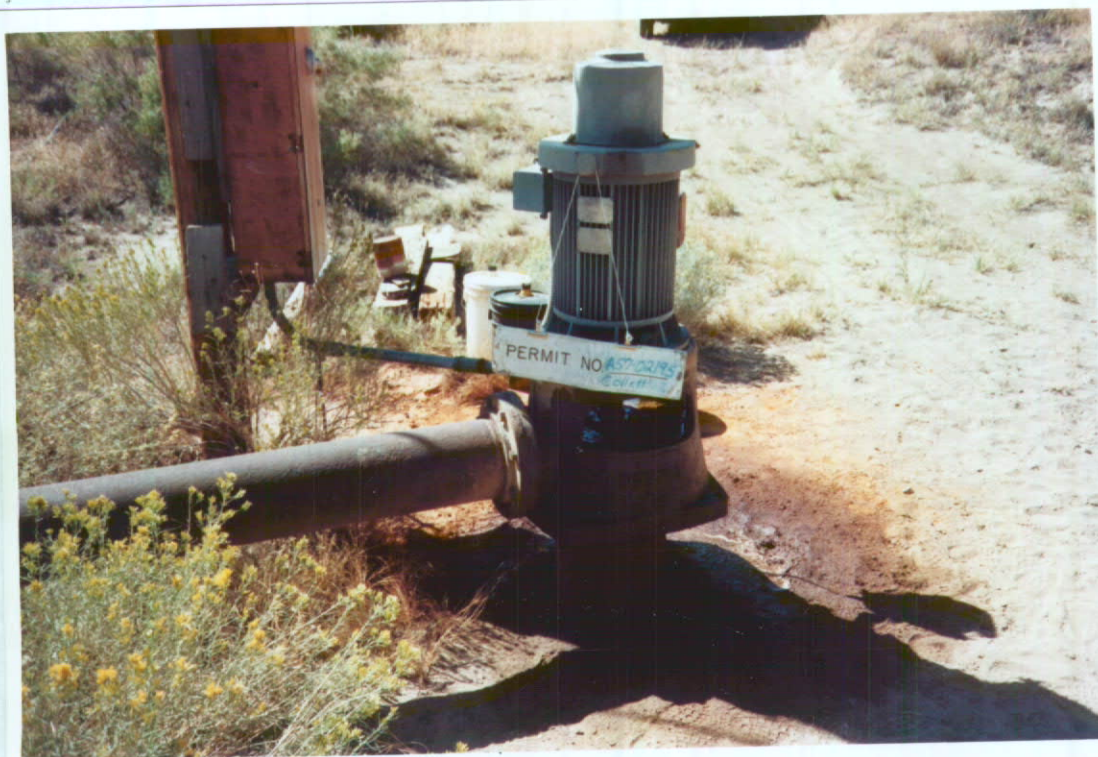
PHOTO ONE- P/O A57-02195 in NESESW S.16 just east of access Road. 8" mainline discharges into cement ditch (photo #2).
