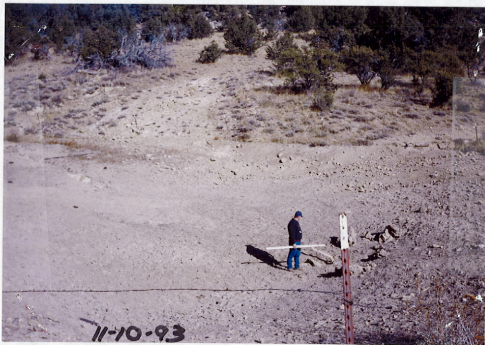
Pond no. 3 (upper one) on Meadow creek. Standing at outlet pipe.
