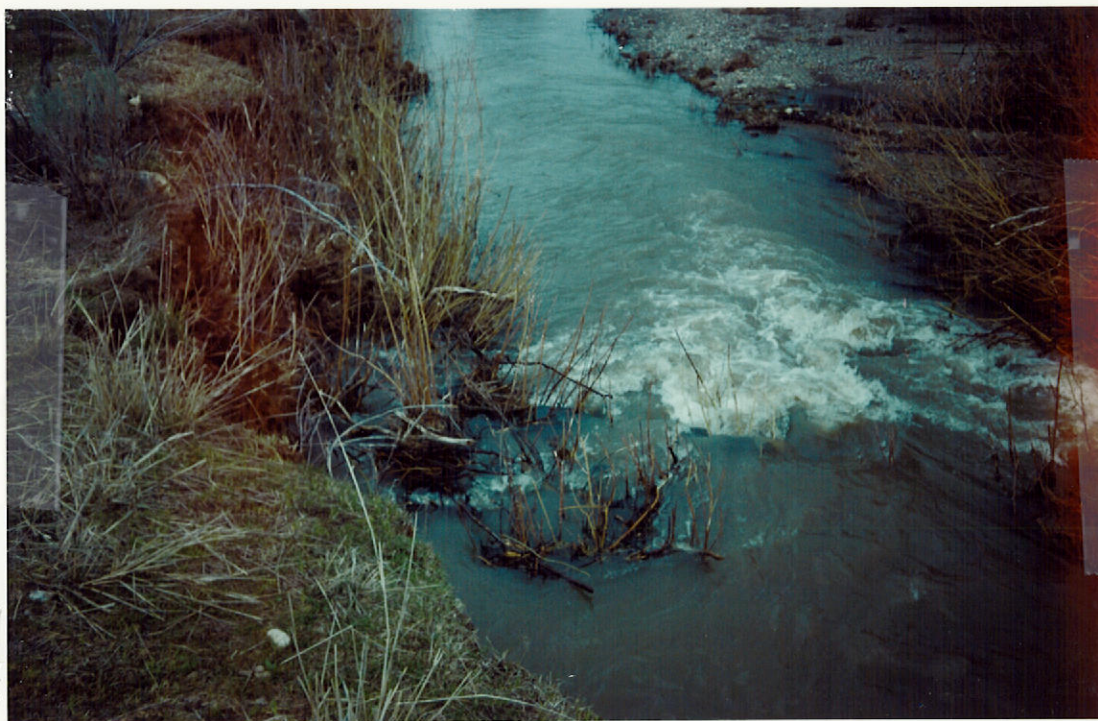
DOWNSTREAM P/D, ROCK DAM, WASHED-OUT.
