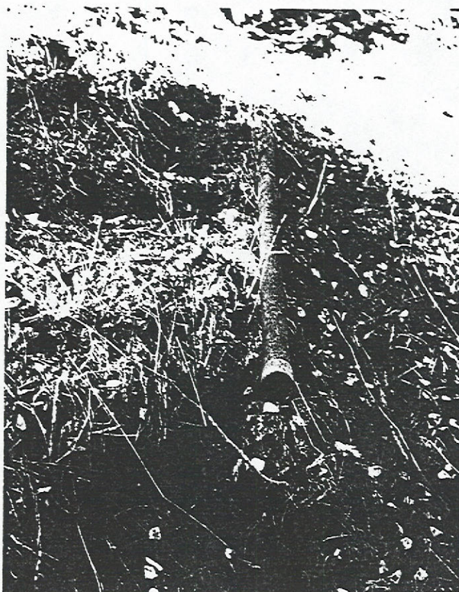
ITEM # 2: Another view of the exposed pipeline of the 1868 Idaho Hotel Spring.
