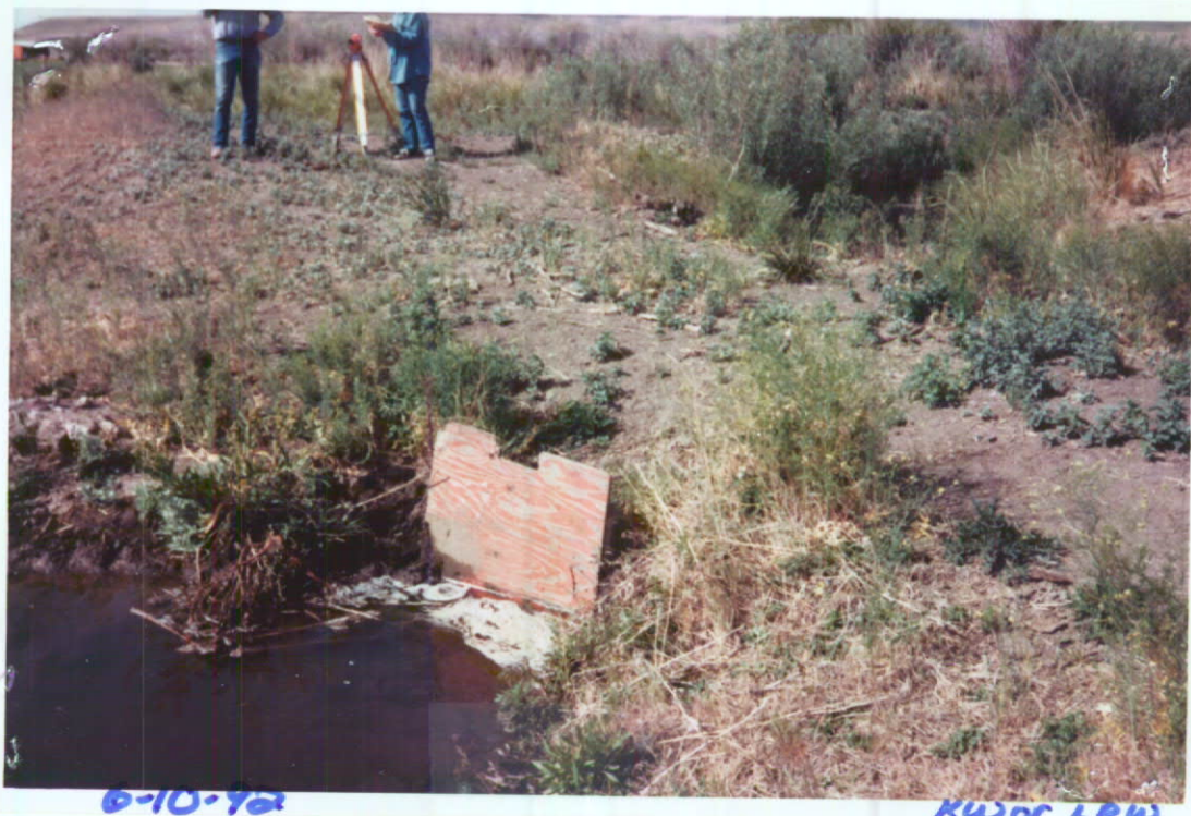
Headgate for POD no. 1 shown above
