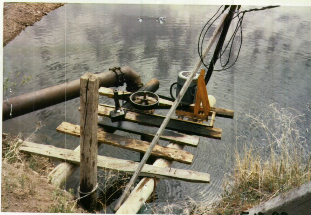
Pump in Jordan cr. Sec. 13, S&SE. Irr. land on west side of creek.
