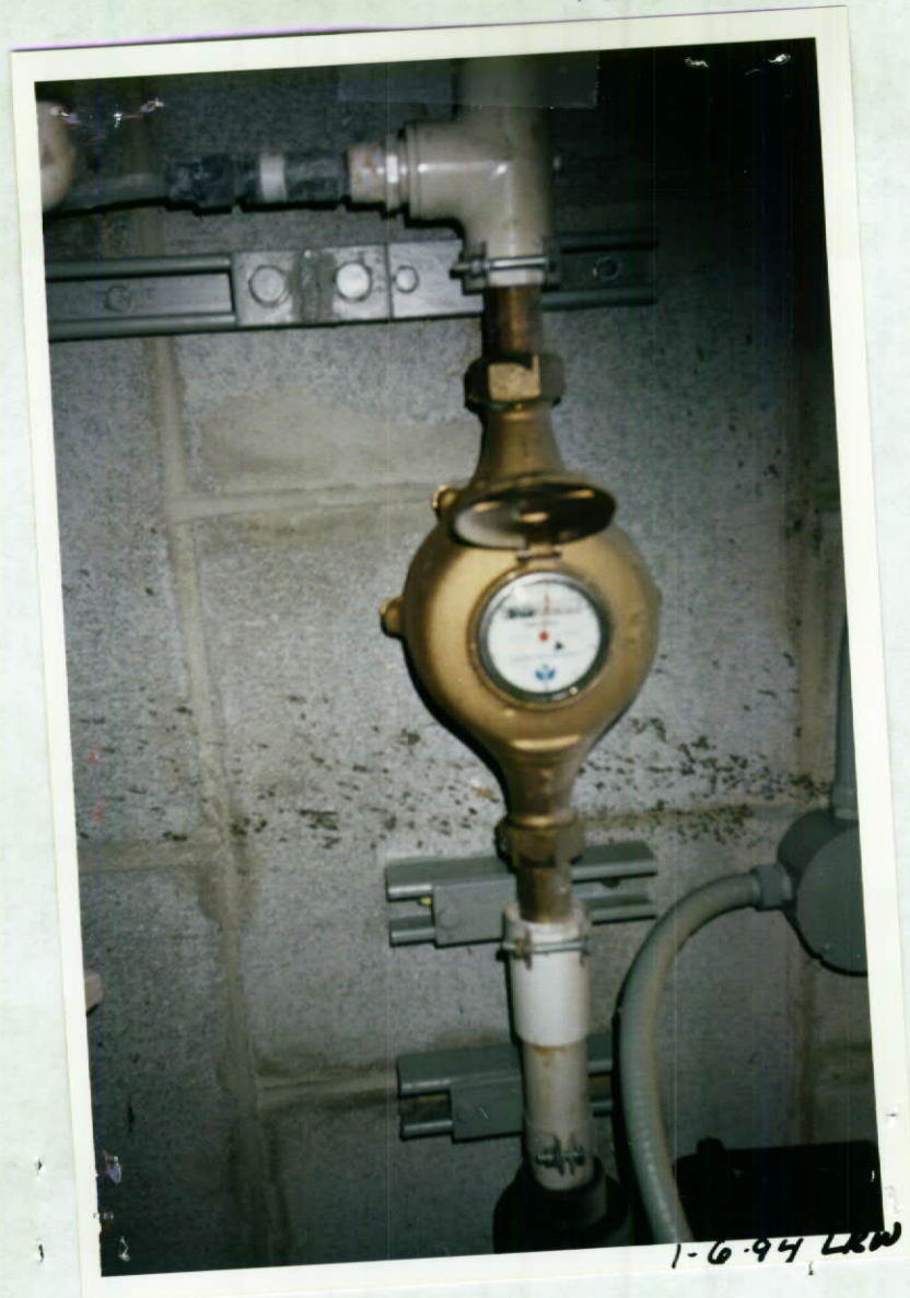
Water meter at fluoridation unit.
