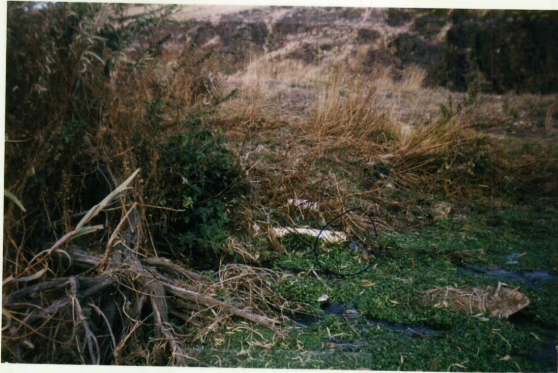
① PVC pipe outlet from Spring Discharges to natural channel.
