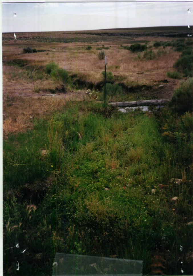
POD, in need of being fixed. Point being recommended.
