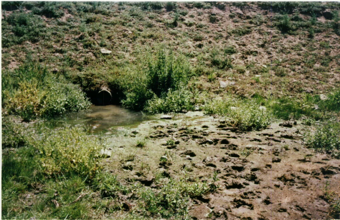
Pipeline from Crawfish Spring pond
