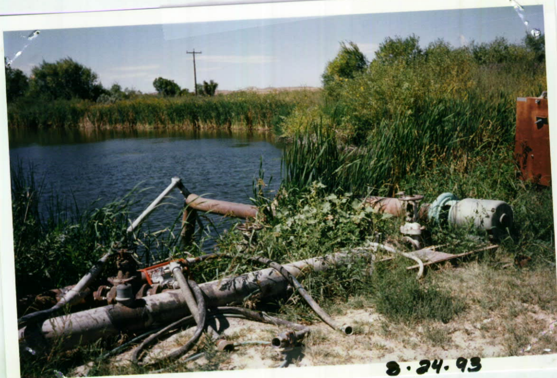
Relift pond w/ 2 pumps - 25 + 40 hp.
